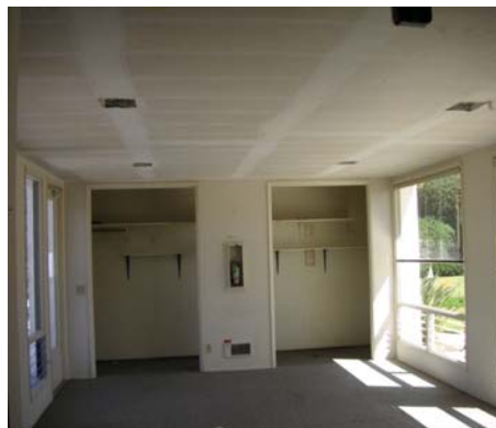
The old clubhouse ceiling is gone.
